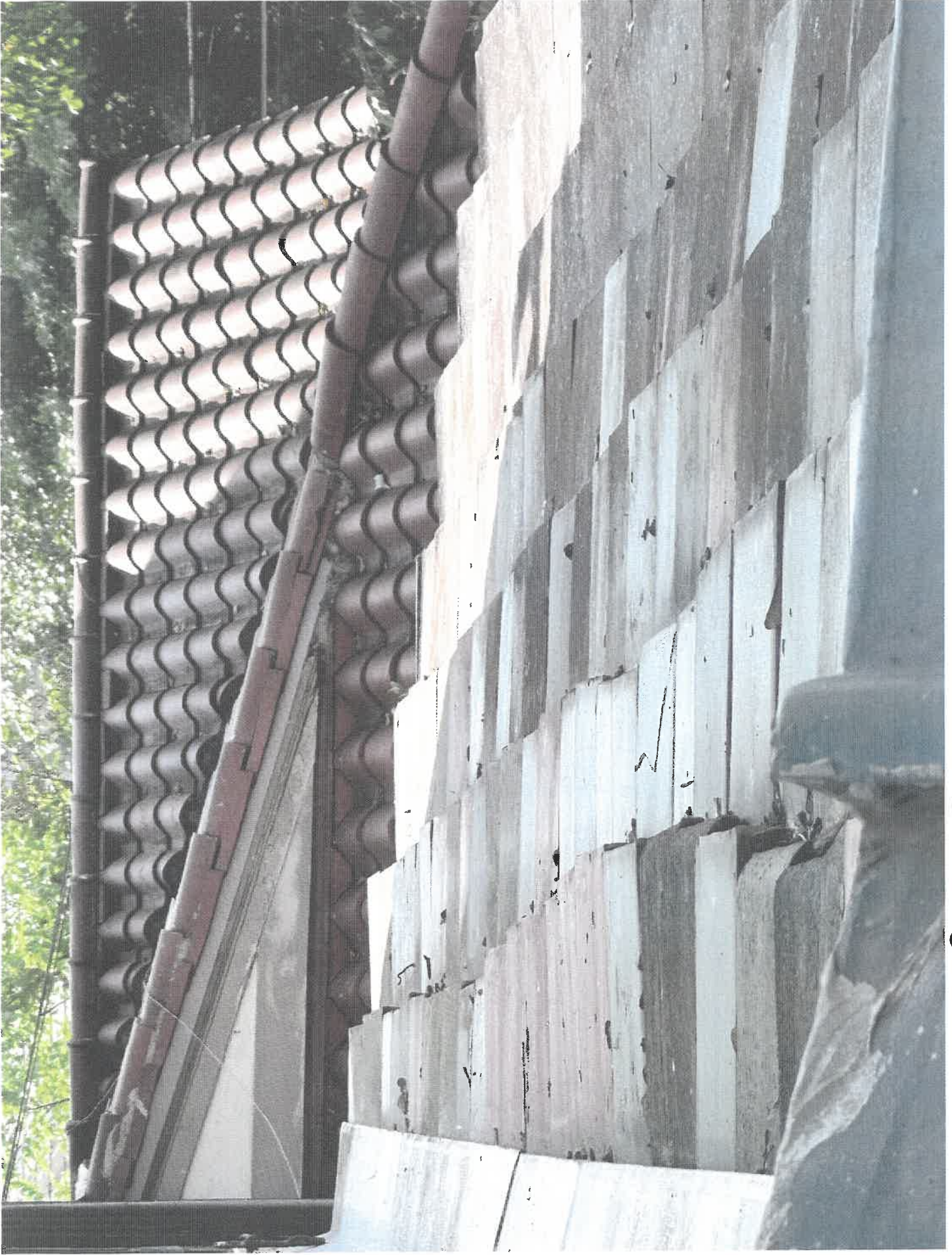
PORCH LEFT SIDE ROOF TILES
