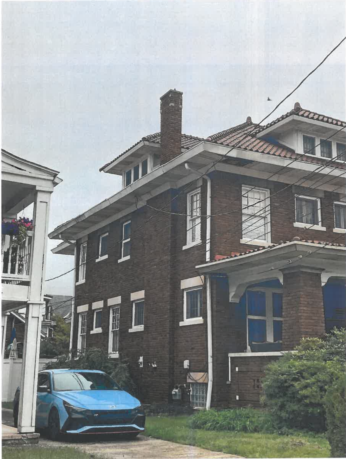
Side view of 1628 Virginia St. E. Damaged soffits in upper corner.
