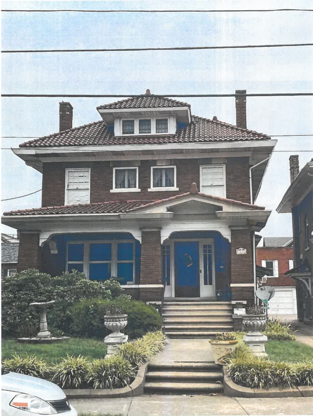
Front view of house, 1628 Virginia St. E. Damaged soffits on upper left corner and lower right corner of porch.
