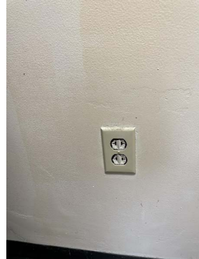
Receptacle (No Ground)
