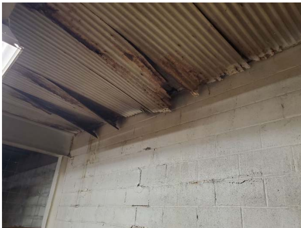
Metal Form Deck and Slab Failure
