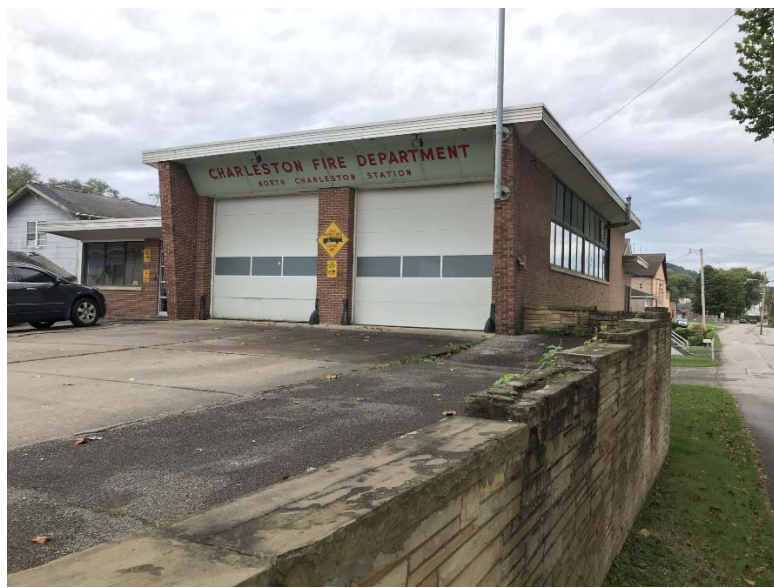
Failing Exterior Retaining Wall
