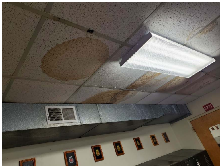
Water Damaged Ceiling Tile
