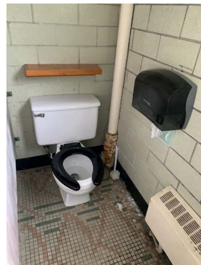
Existing Tank Type Toilet
