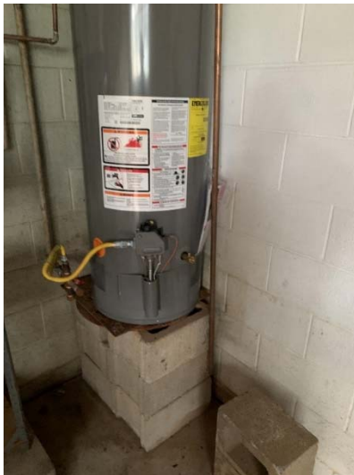
Existing Water Heater
