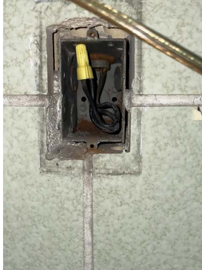
Open Junction Box
