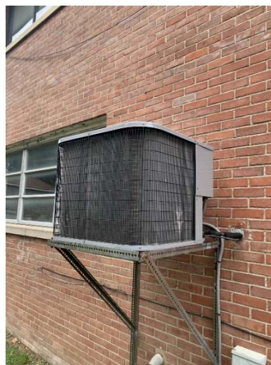
Raised Condensing Unit
