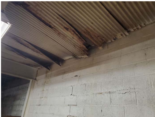
Metal Form Deck and Slab Failure
