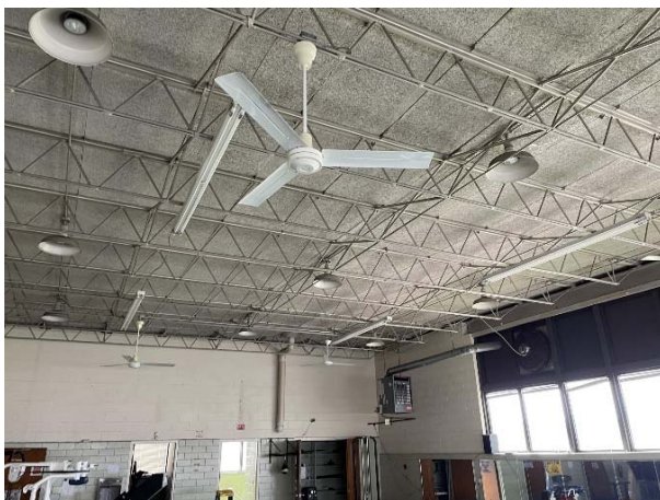
Fitness Area Lighting
