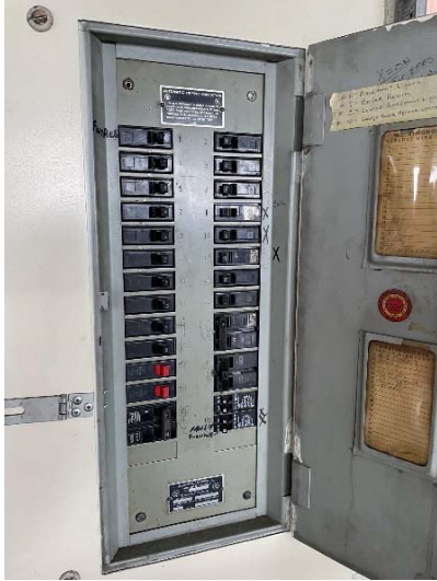
Existing Electrical Panel
