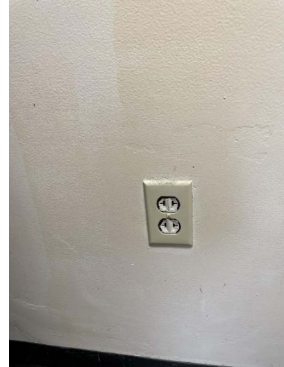
Receptacle (No Ground)
