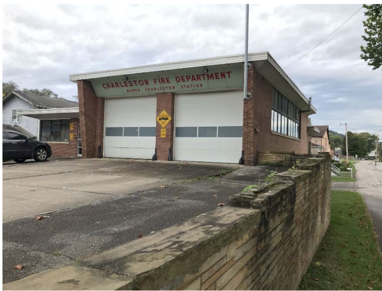
Failing Exterior Retaining Wall
