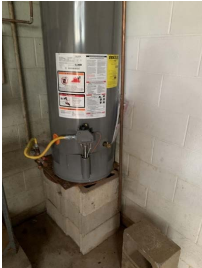
Existing Water Heater
