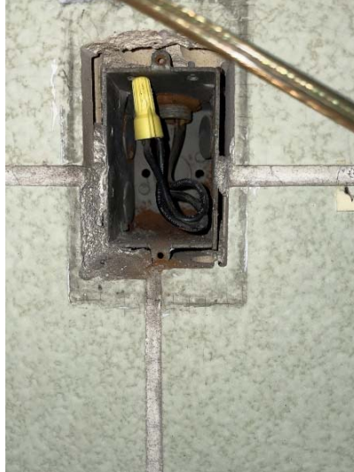
Open Junction Box
