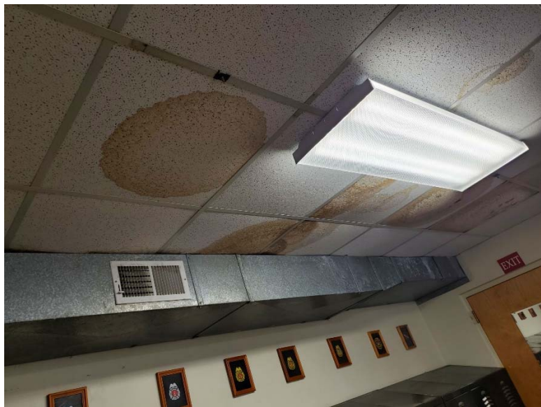
Water Damaged Ceiling Tile
