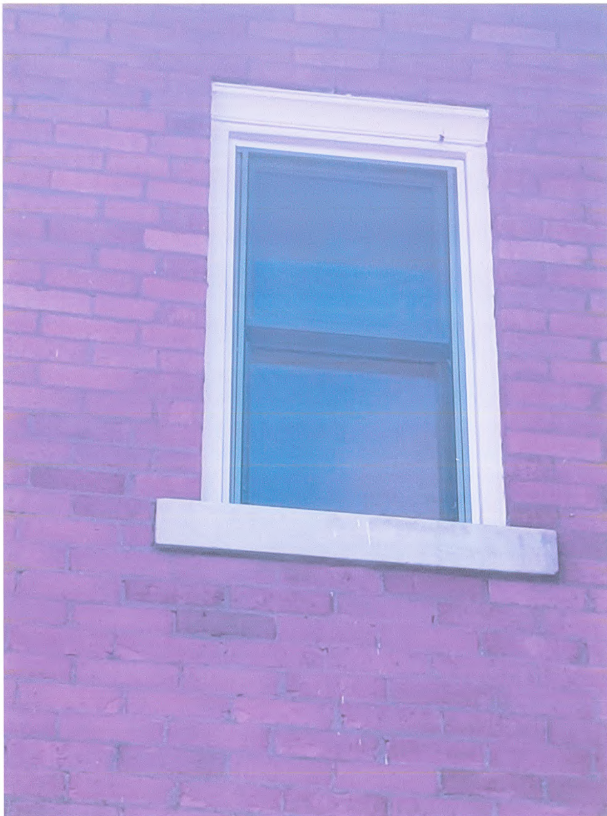
Exterior view of Pella double hung architect window replaced in 2015.
