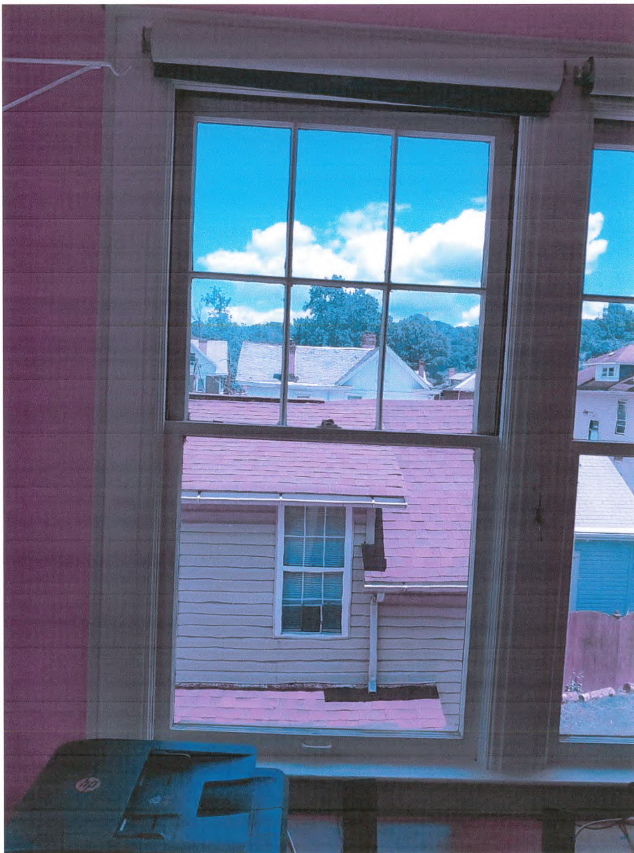
1 of 4 north facing sleeper porch windows. Window does not open. No bug screen.
