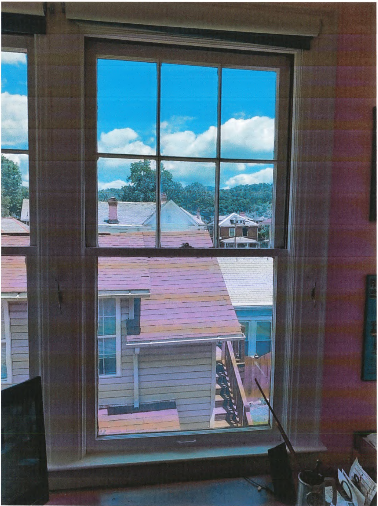
2 of 4 north facing sleeping porch window. Lower pane is plastic, and it rattles in high wind.
