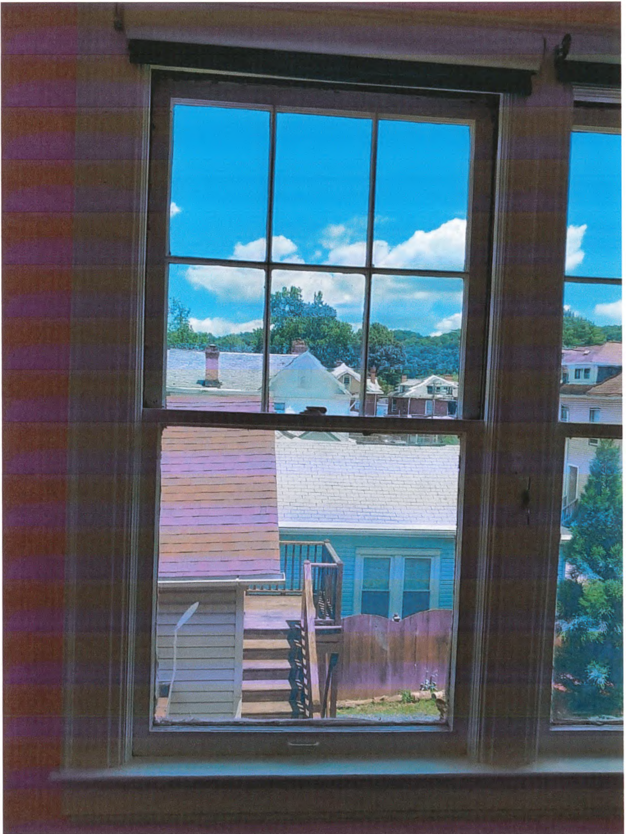
3 of 4 north facing sleeping porch windows. Lower pane is plastic, and it rattles in the wind.
